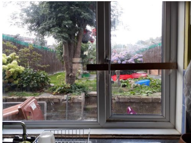
Photo 4: Damaged kitchen window
