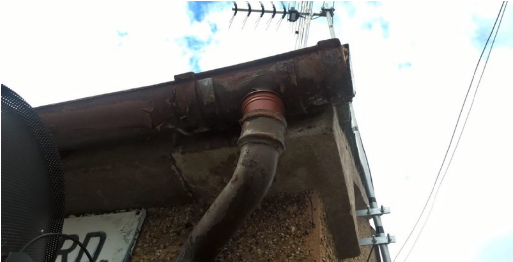
Photo 1: Plant pot holding guttering together at living-room corner
