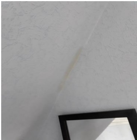
Photo 3: Damp on upstairs bedroom ceiling
