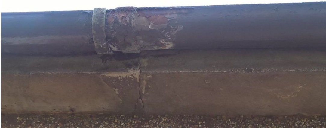
Photo 2: Broken guttering and cracked masonry at bedroom corner
