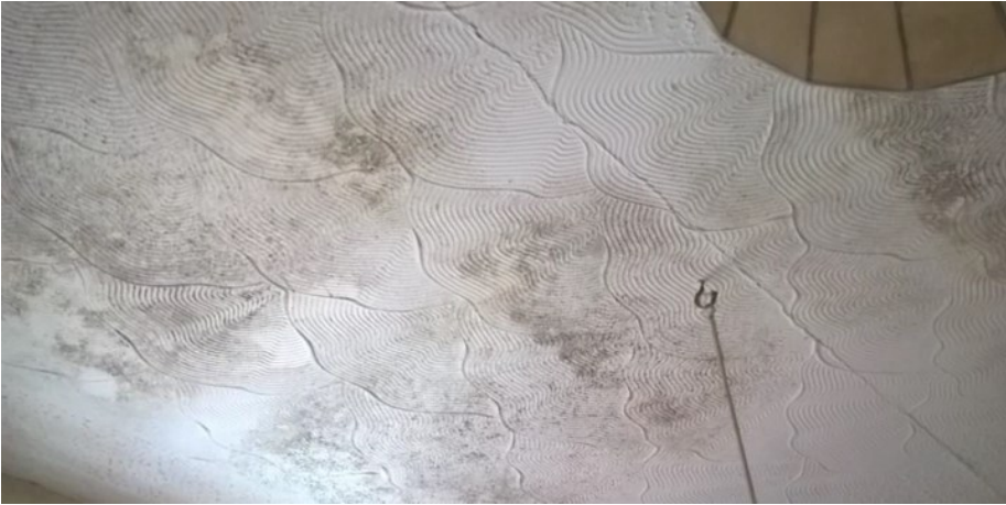
Photo 1: Mould on kitchen ceiling under flat roof
