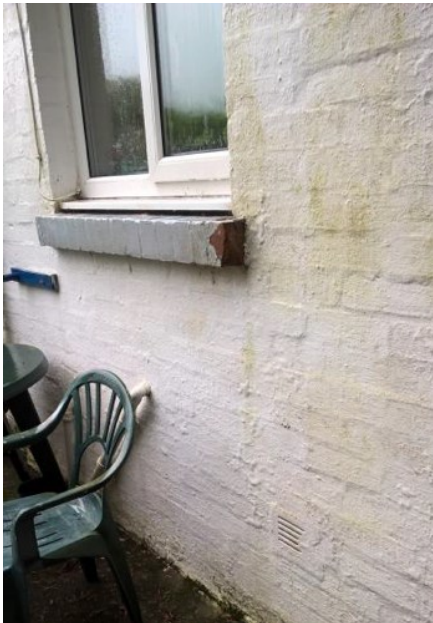
Photo 3: Extension wall construction showing thickness of wall. Condensation is visible on inside of kitchen window.
