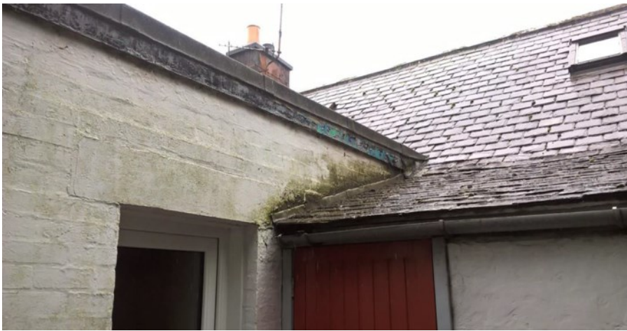
Photo 2: Flat roof to extension, join of pitched roof to extension (kitchen door)
