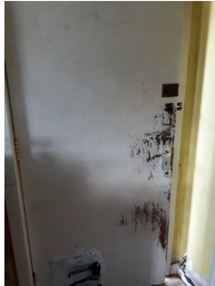
Photo 2: interior door used for exterior door
