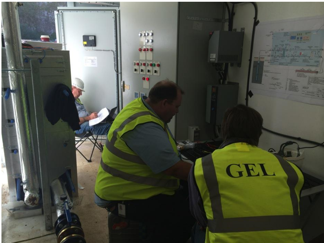
Figure 18 Thermal Response Test unit showing heat exchanger and central control panel
