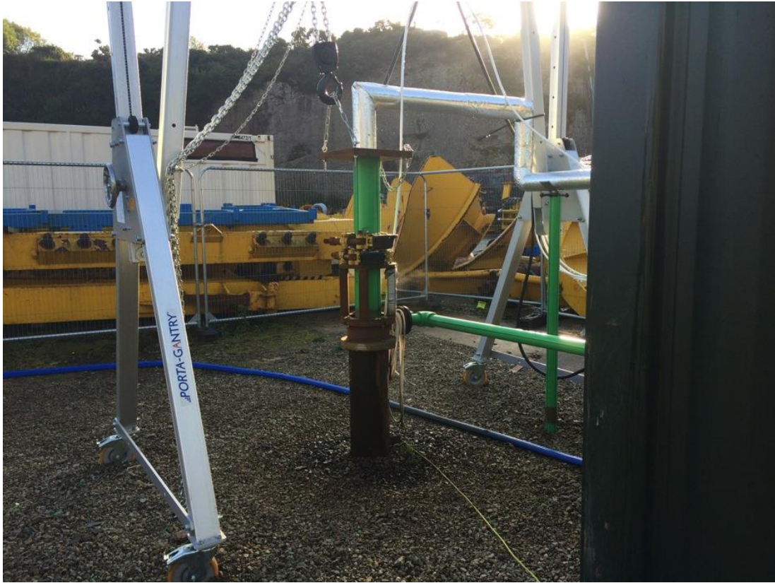
Figure 16 Completed well-head connections to the Thermal Response Test unit
