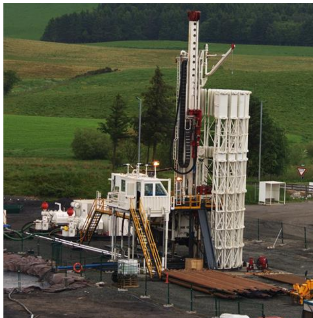
Figure 15 Example of the Drillemec HH102 that we propose to use at the AECC site
