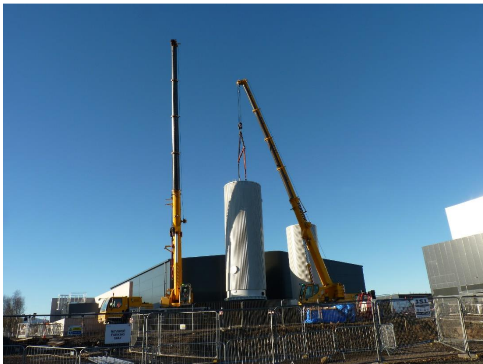
Figure 10. Energy centre for the Millerhill Low Carbon District Heating Project (© Vattenfall)
