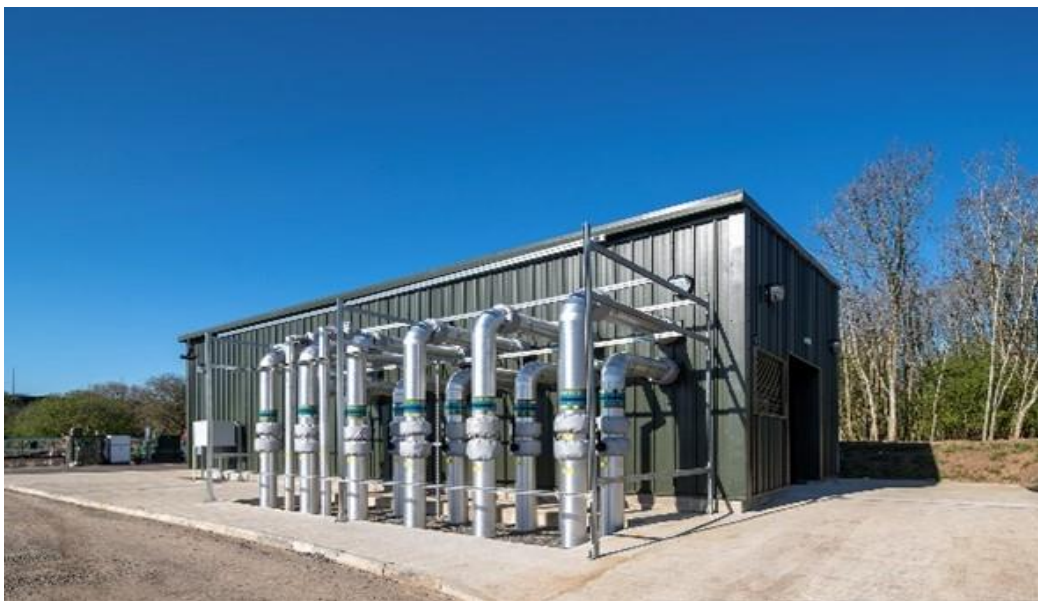
Figure 5. Energy Centre at AMIDS heat network (© Paul Zanre)
