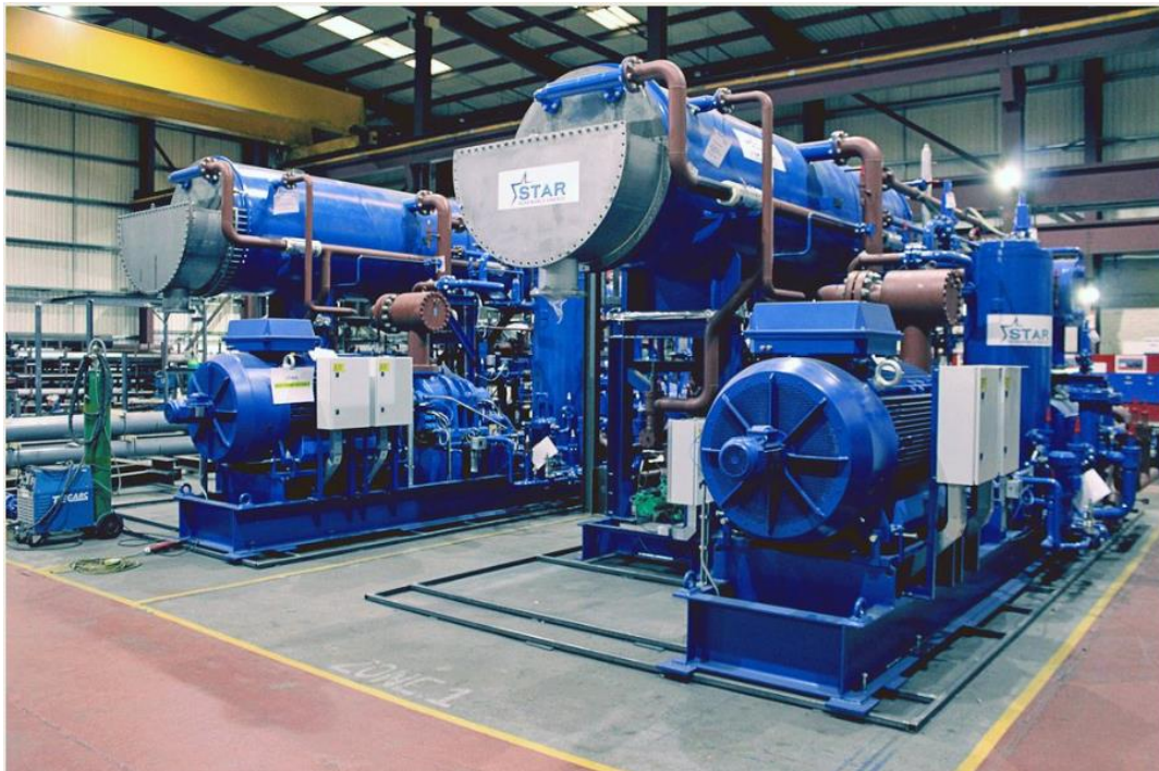
Figure 20. Queen's Quay Energy Centre (Credit: West Dunbartonshire Council)
