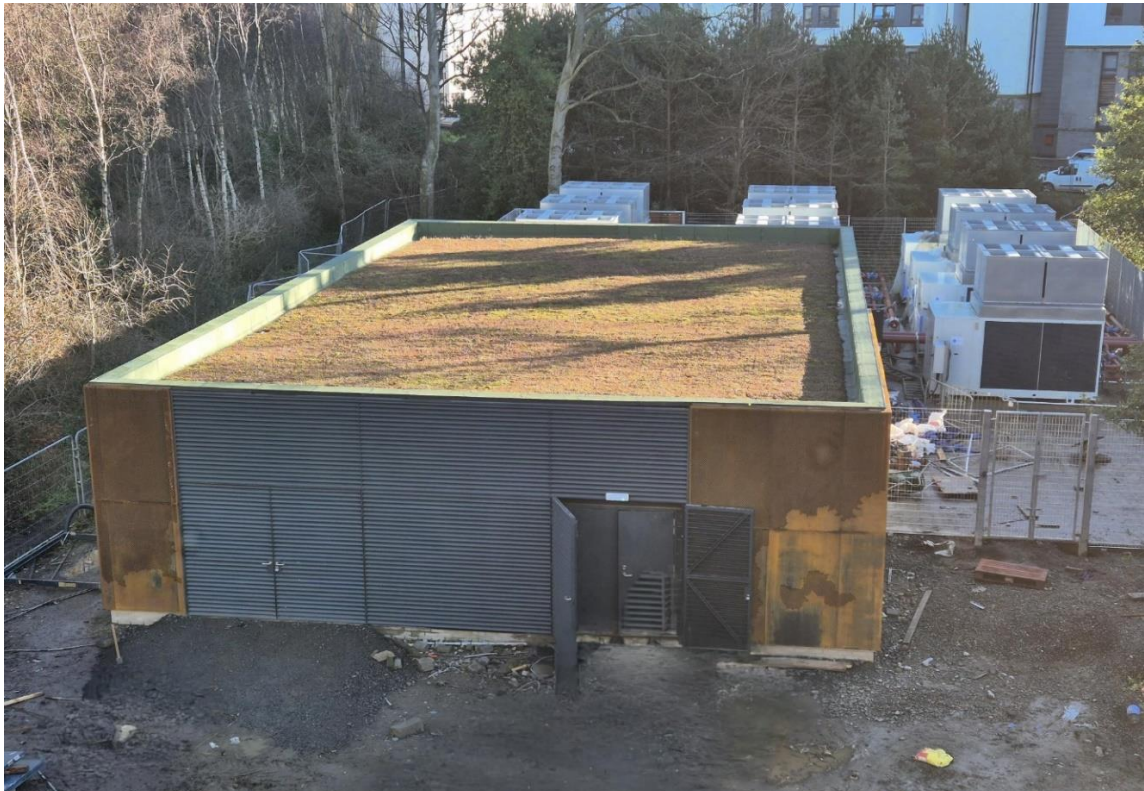
Figure 11. Image of the energy centre with ASHPs at Western Villages site (© City of Edinburgh Council)
