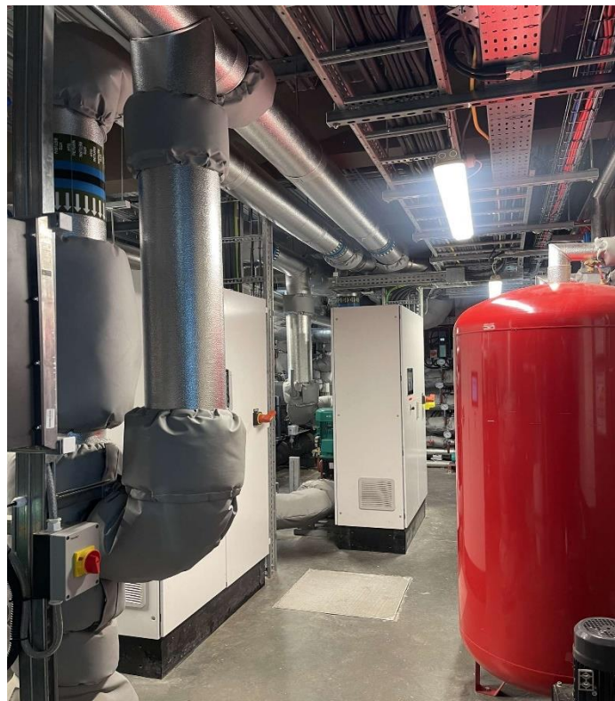
Figure 9. Glen Mhor Energy Centre (© Glen Mhor Hotel)
