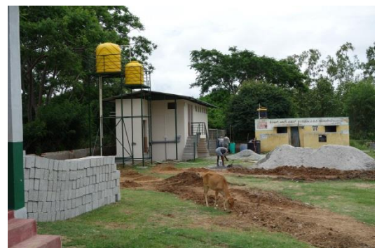
Image: New toilet block (left) and the old toilet block to the right
